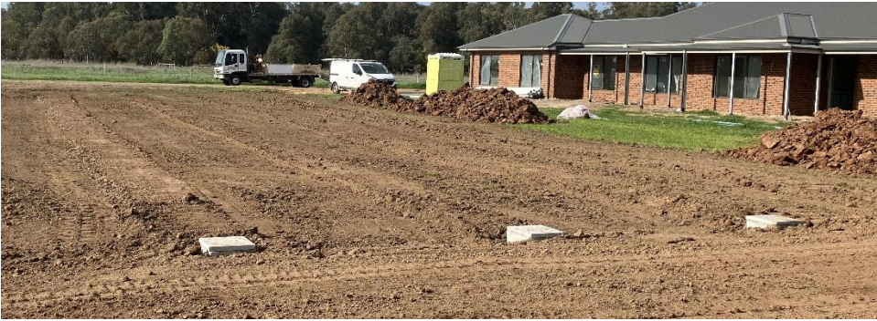
Image 16: Completed work – top of each trench is domed above natural ground so that surface water/rain does not sit on top of the trenches.
