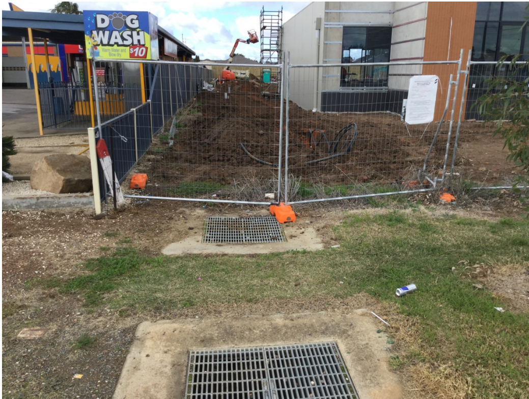
Two existing pits that need to be incorporated into any vehicle access
