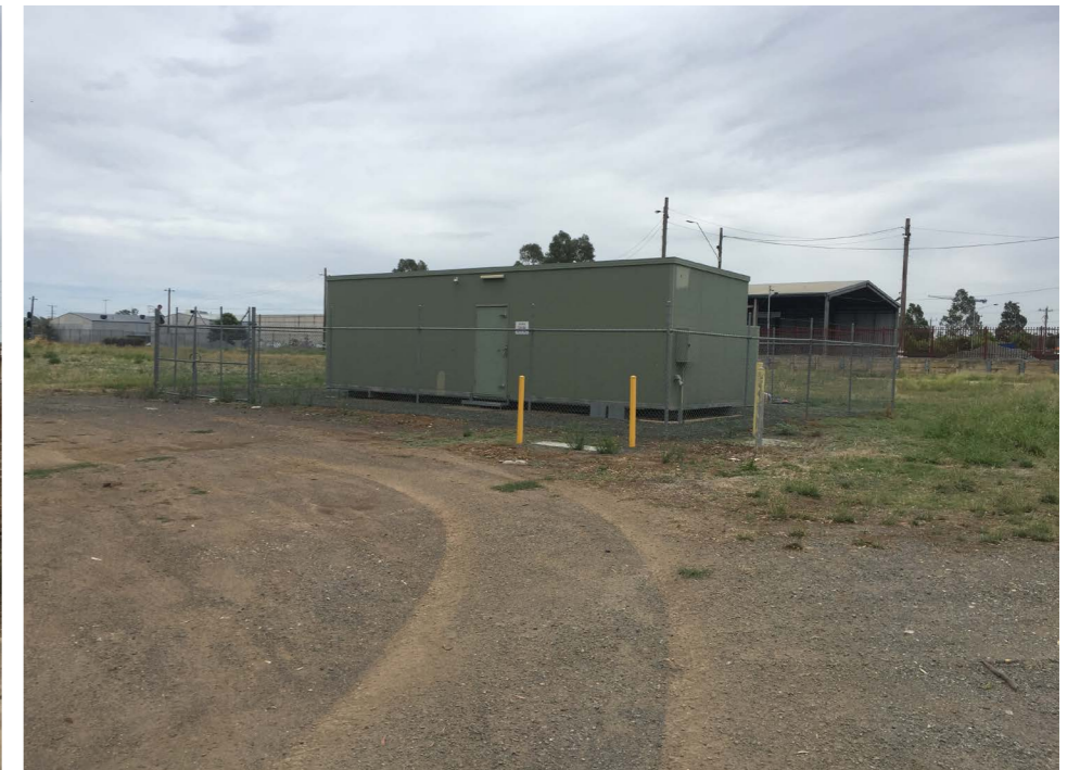
Figure 15 Building No.20 High security fenced and windowless electrical substation off Purcell Street (for supplying V/Line signaling power)
