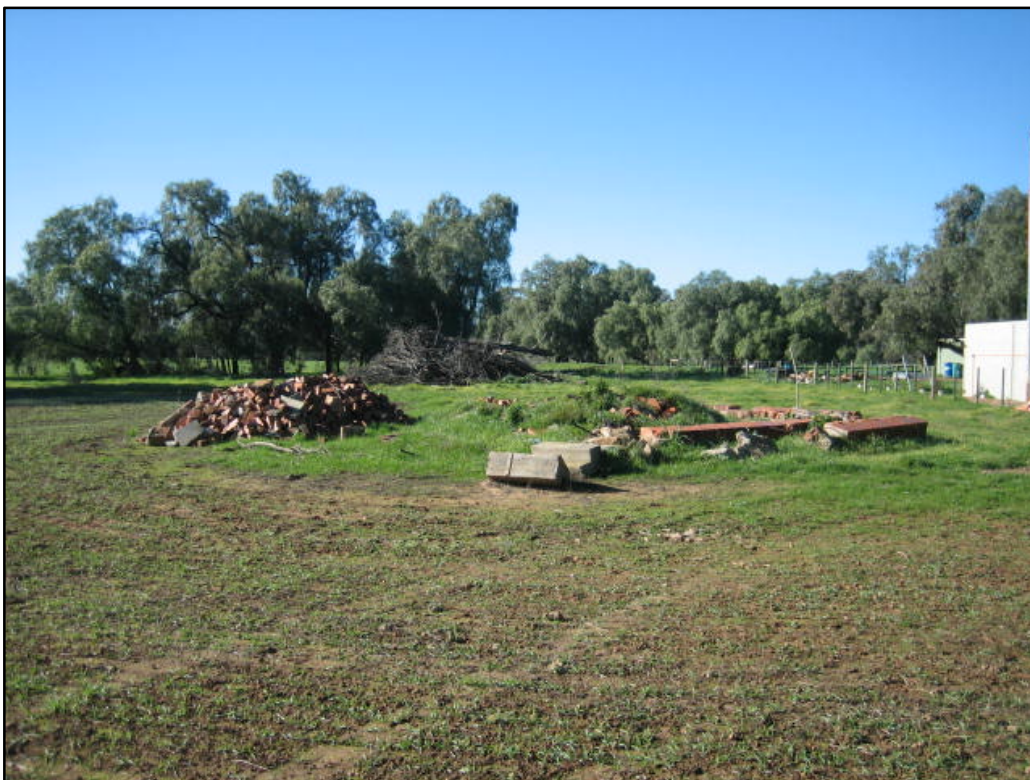
Plate 4: View of a stockpile of demolition waste observed on the southern portion of the site. Some evidence of burning of materials was also noted at this location. The structure on the right of the photo is a shed associated with the on-site dwelling.
