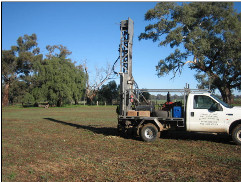
Plate 6: View of drilling works in progress on the southern portion of the subject site. Drilling was completed with a rotary auger drill rig operated by Llyod Angove Soil Surveying & Drilling.
